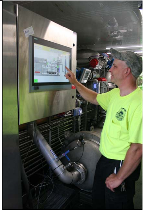
Park Ridge Water Department Operator Mark Gronbeck operating the controls on the new Purifics photo-catalytic advanced oxidation treatment system at Well 17.
